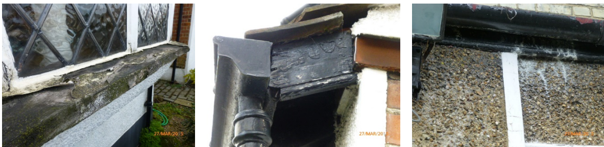
External window frames are poor
