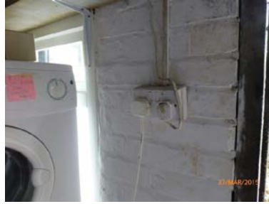
Electrical installation to be checked
