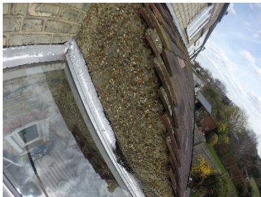
Verge tiling is loose and defective
