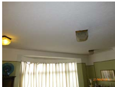
Lights not working
