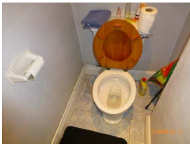
Damp staining to walls
