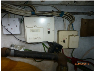
Fuse-board is dated
