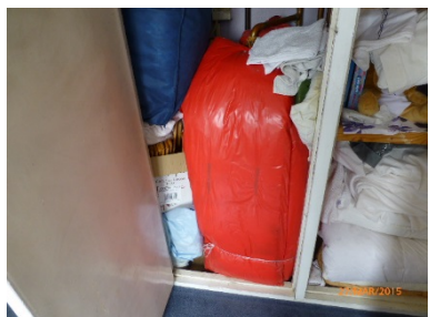
Unlagged hot water cylinder
