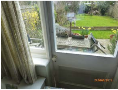
Glass in a critical location
