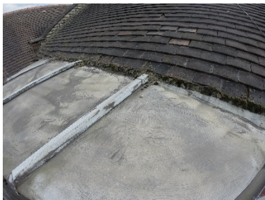
Front bay window roof is worn
