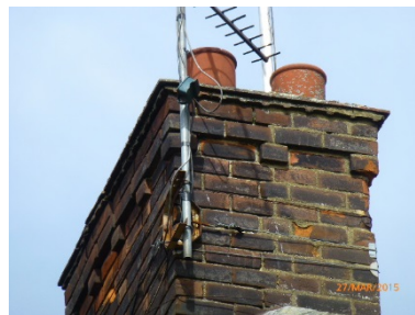
Spalled bricks and loose pointing
