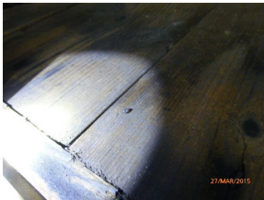
Rodent droppings in the roof space
