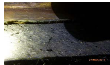
Some evidence of wood boring insect
