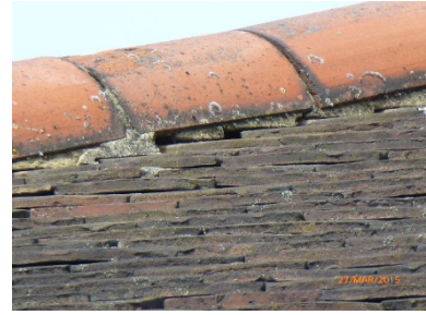
Mortar to the hip/ridge tiles is poor
