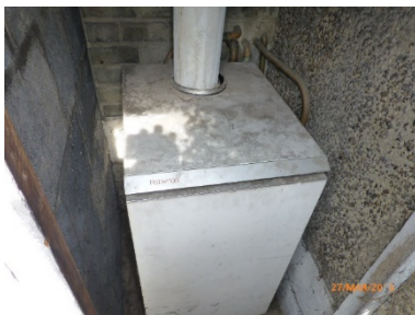
Floor standing boiler
