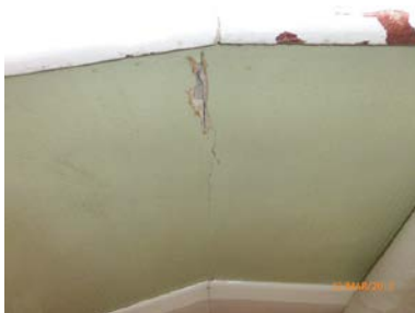
Small crack to front bay
