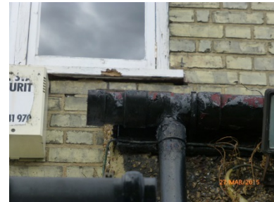
Decoration to rear gutters is poor
