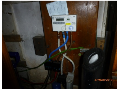
Main fuse and meter
