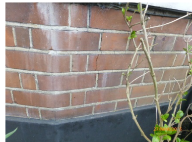
Crack to the left side of the bay
