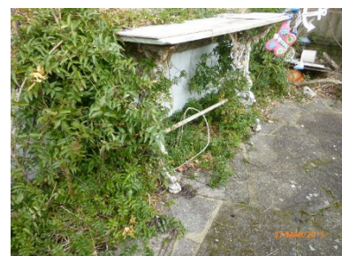
No air bricks to the rear
