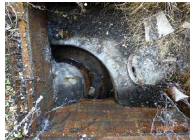
Inspection chamber is dirty
