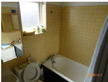
Installation is dated
