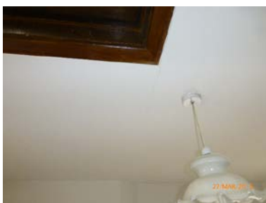
Crack to landing ceiling
