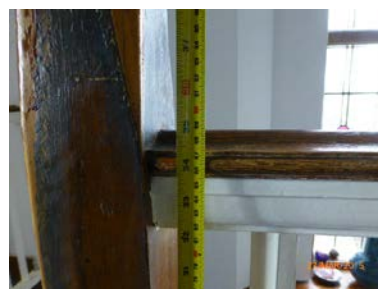
Landing hand rails are low
