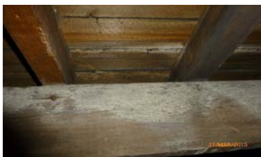
White spores to the roof timbers
