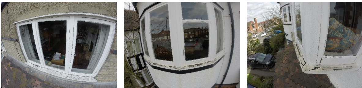
Window frames are in a poor state of repair
