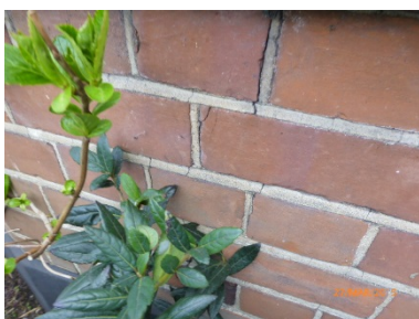
Crack to the centre of the bay
